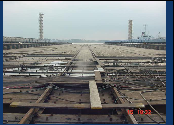
Picture showing timber Sleepers removed exposing both Main Transverse and Intermediate Transverse Beams. Date of work commencement 15 th March 2002
