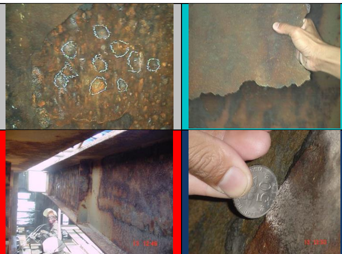
Pictures showing initial substrate conditions with heavy pitting original coating delaminating. Date of Work commencement 15 th March 2002
