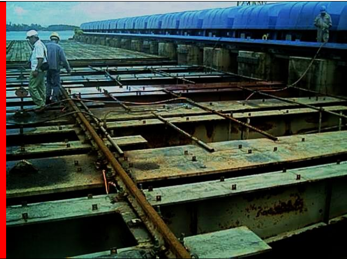
Picture showing timber Sleepers removed exposing both Main Transverse and Intermediate Transverse Beams. Date of work commencement 15 th March 2002
